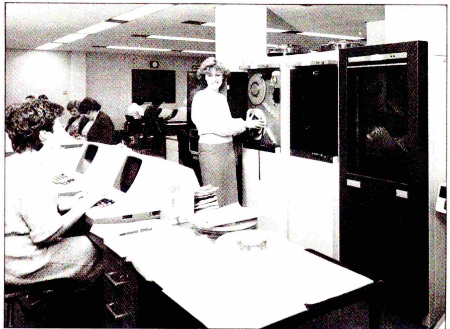
Three Rediffusion BCGs are installed on the first floor of the data preparation centre at Centre-file Romford
